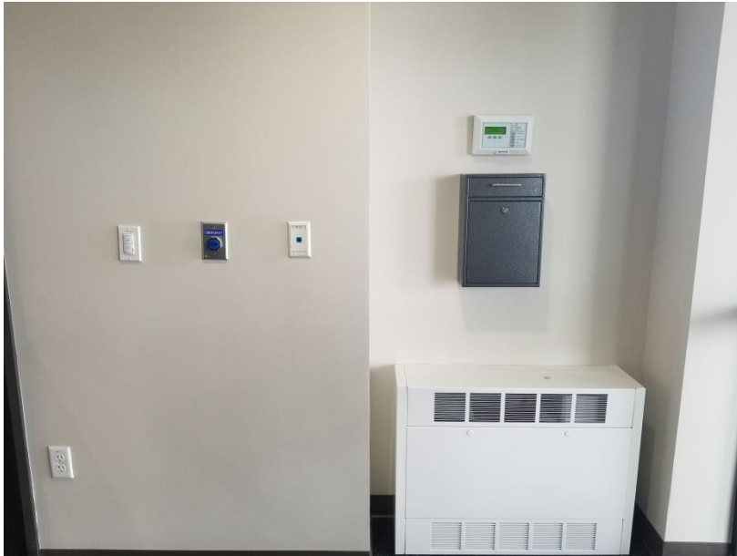
SECURE AFTER HOURS VESTIBULE
