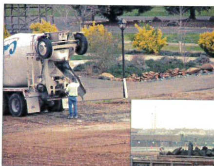
Figure 1. Chute washwater being dumped on the ground
