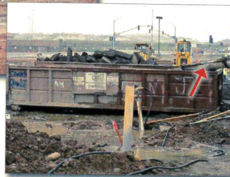
Figure 2. Chute washwater leaking from a roll-off bin being used as a washout container
